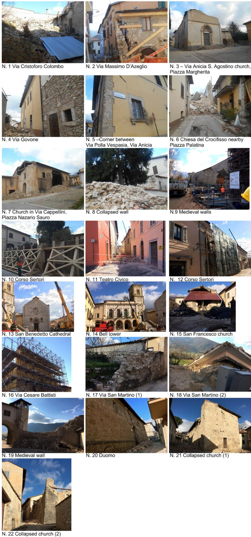
Figure S6. Pictures of all structures with assigned damage level D5 in the city center of Norcia, along with their identification numbers.
