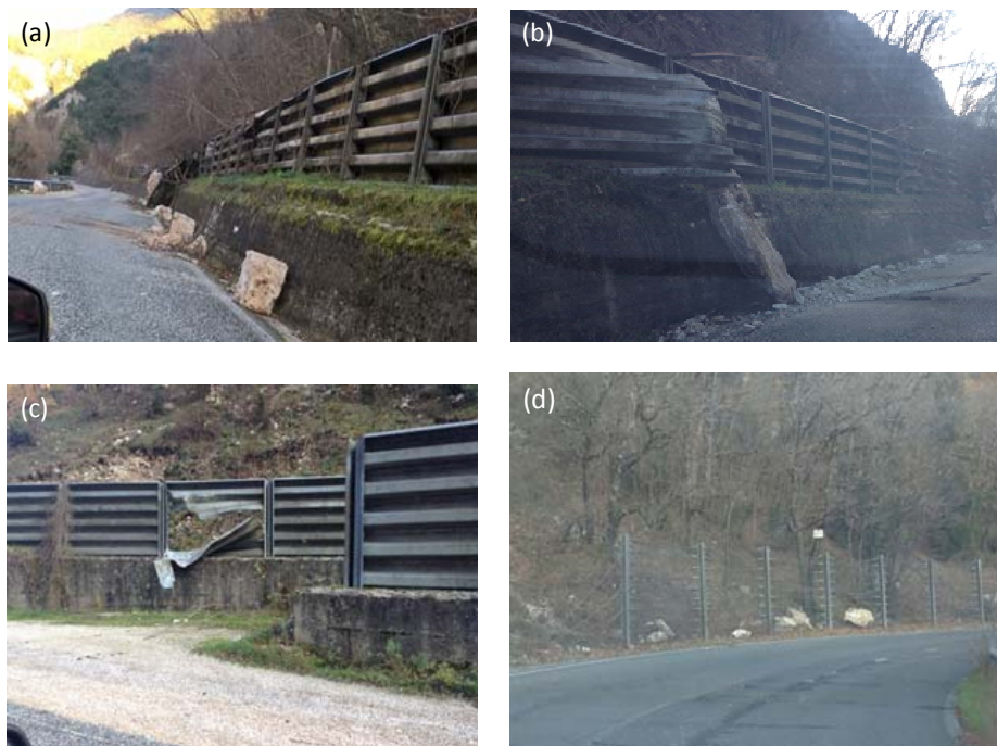
Figure 25: Slope protection damaged by boulders and rock-blocks along the regional road SP 290 in the Nera river valley (adapted from GEER, 2017).
