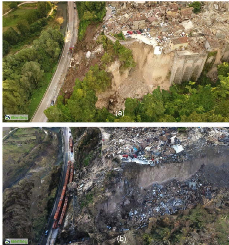
Figure 31: 3D model of the failed retaining wall area in Pescara del Tronto (areas #3-4 in Figure 28) following: (a) the 24 August and (b) the 30 October event (from GEER, 2017).
